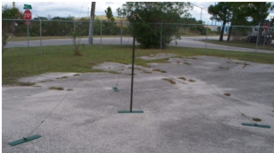
Example: The sand bags must be placed over the two sides of the plates.
